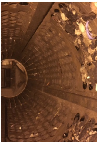
Sections inside the trommel clear of waste where the metal rings have been fitted and clogged holes without external rings.
